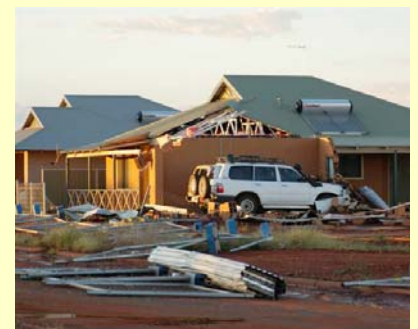
Storm damage ... a GEHA home damaged by a freak storm at Warburton in November 2005.
