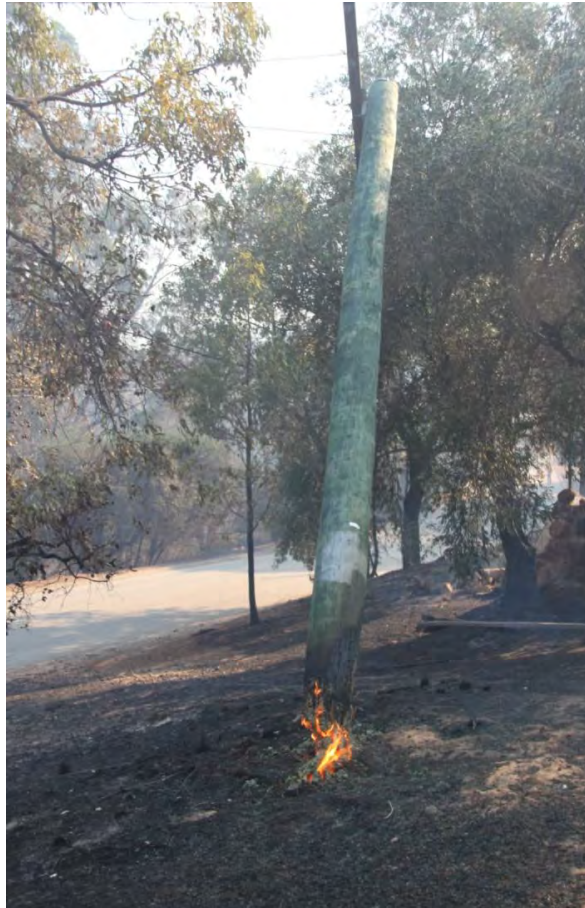
Power pole on fire in Kelmscott – 6 February 2011 228
