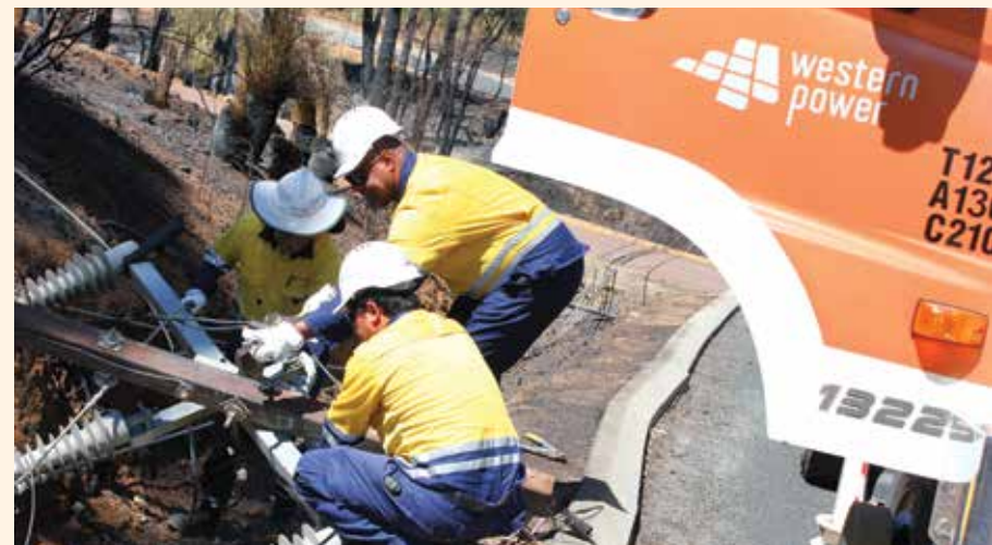
Figure 4.6 – Western Power crews assessing damage to their infrastructure following the Parkerville Stoneville Mt Helena Bushfires in January 2014
