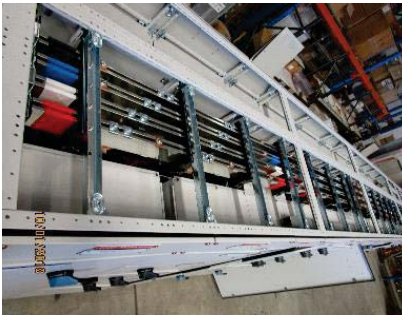
Centre fed MCC busbar system. The standard CUBIC busbar system was designed as ring busbar system for back to back MCCs. We worked with NHP and designed a center fed busbar system with horizontal main bus and front and back common dropper. This saves significant amount of copper.
