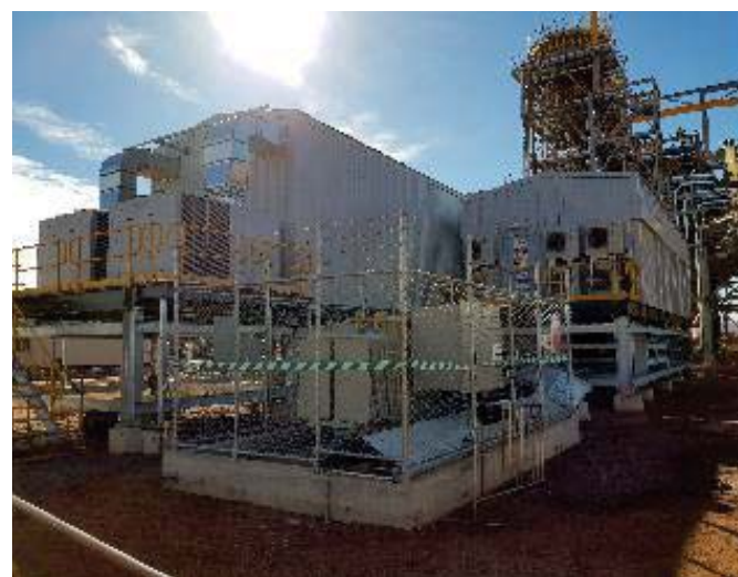
Installed switchroom Pilgangoora Lithium project
