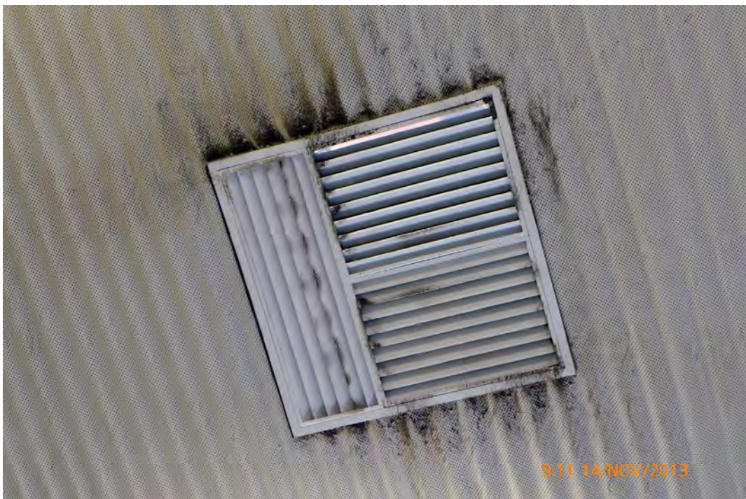
Figure 9: The dusty air conditioning units in the accommodation blocks
